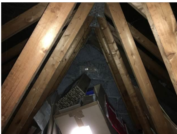
Photograph 5: Showing the interior of the loft space of the main structure (Section A)
