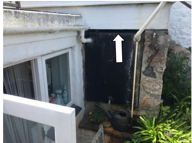
Photograph 4: Showing the integral water tank beneath the conservatory. The gap at the top providing access to the location where a historic nest was confirmed can be seen.
