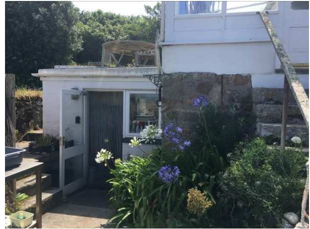
Photograph 2: Showing the conservatory (Section B) built on top of the flat-roof extension (Section C)
