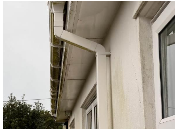
Photo 14 - Showing a closeup of the soffits which run around the hospital building (B6) - these are well sealed throughout.
