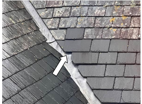
Photo 12 - Showing an example of the minor lifted tiles present around the valley where roof pitches join on the hospital building (B6)
