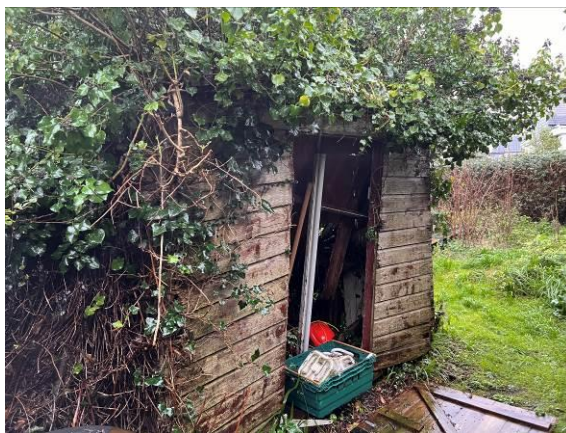
Photo 19 - Showing the derelict wooden shed (B5) which is overgrown with ivy and the roof inside has collapsed - the potential access for bats can be seen through the open door.
