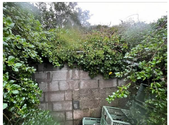
Photo 20 - Showing the derelict outbuilding (B4) which is overgrown with ivy.
