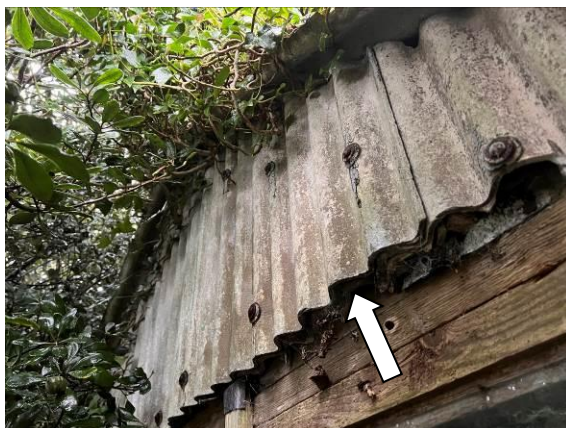
Photo 21 - Showing the corrugated sheeting on the derelict outbuilding (B4) which could potentially provide access to roosting opportunities.
