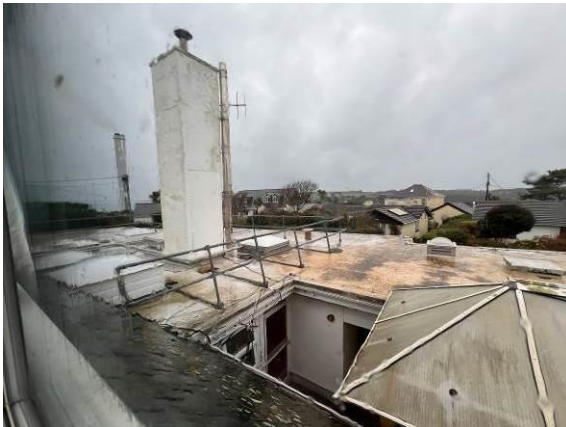
Photo 13 - Showing the flat roof components of the hospital building (B6) which are not considered to offer roosting opportunities for bats.
