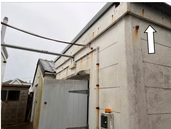
Photo 15 - Showing the emergency generator shed (B9) with gaps around the fascia board which could potentially offer roosting opportunities.
