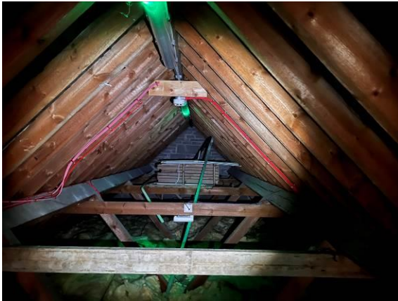
Photo 11 - Showing the interior of a loft space within the main hospital building (B6) with a large void, timber frames and utilities/services running through.
