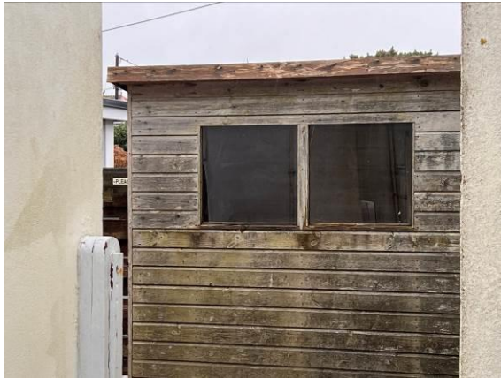
Photo 17 - Showing the garden shed (B10) which is considered to have negligible potential for roosting bats.
