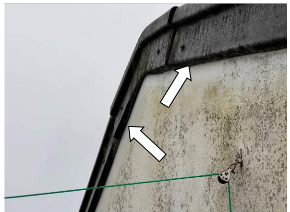
Photo 16 - Showing the apex of the outdoor store room (B7) with gaps behind the gable capping which could potentially permit access to the building and the wall plate.
