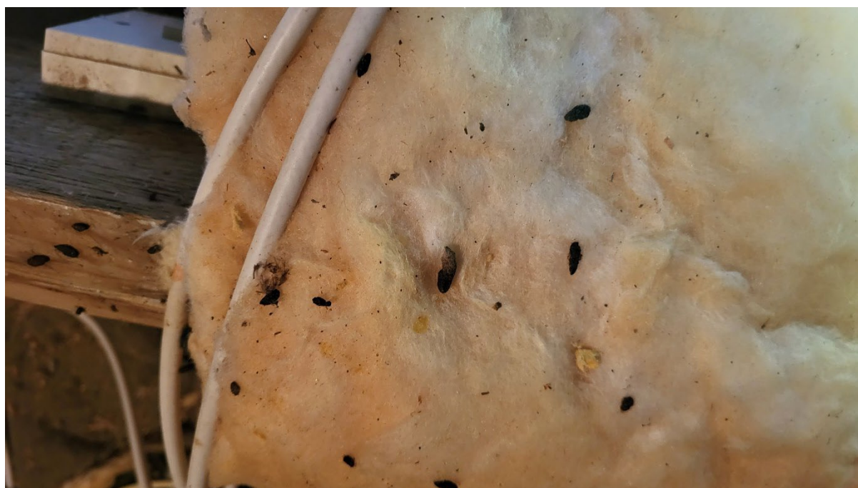
Figure 21: Droppings in the roof void at Racket Town
