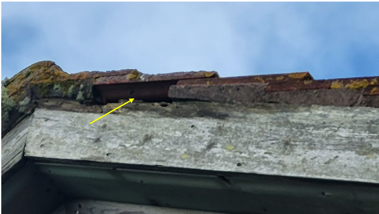
Figure 15: Gap beneath roof tile on the south elevation (yellow arrow)
