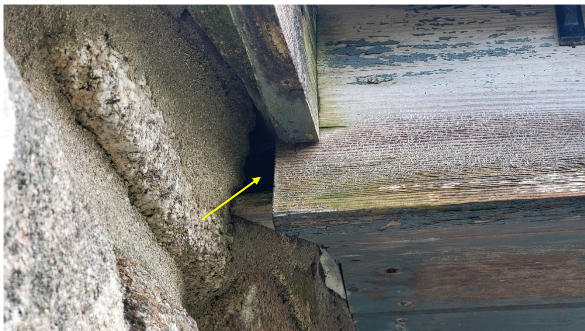
Figure 12: Gap between timber fascia board and the wall at the porch (yellow arrow)
