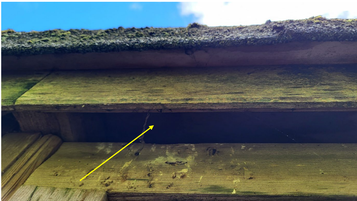
Figure 19: Gap between timbers allow access into the boiler room on the north elevation (yellow arrow)
