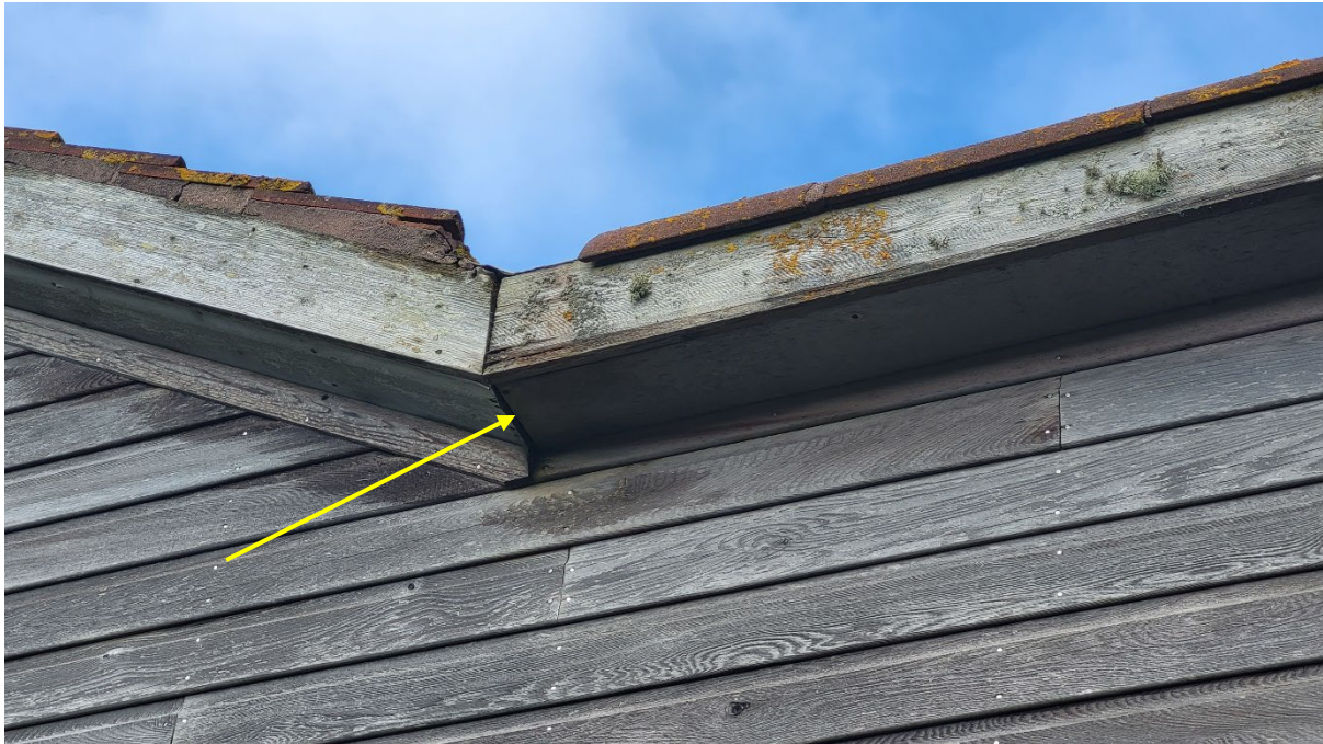
Figure 14: Gaps between fascia boards and soffit on the south elevation (yellow arrow)
