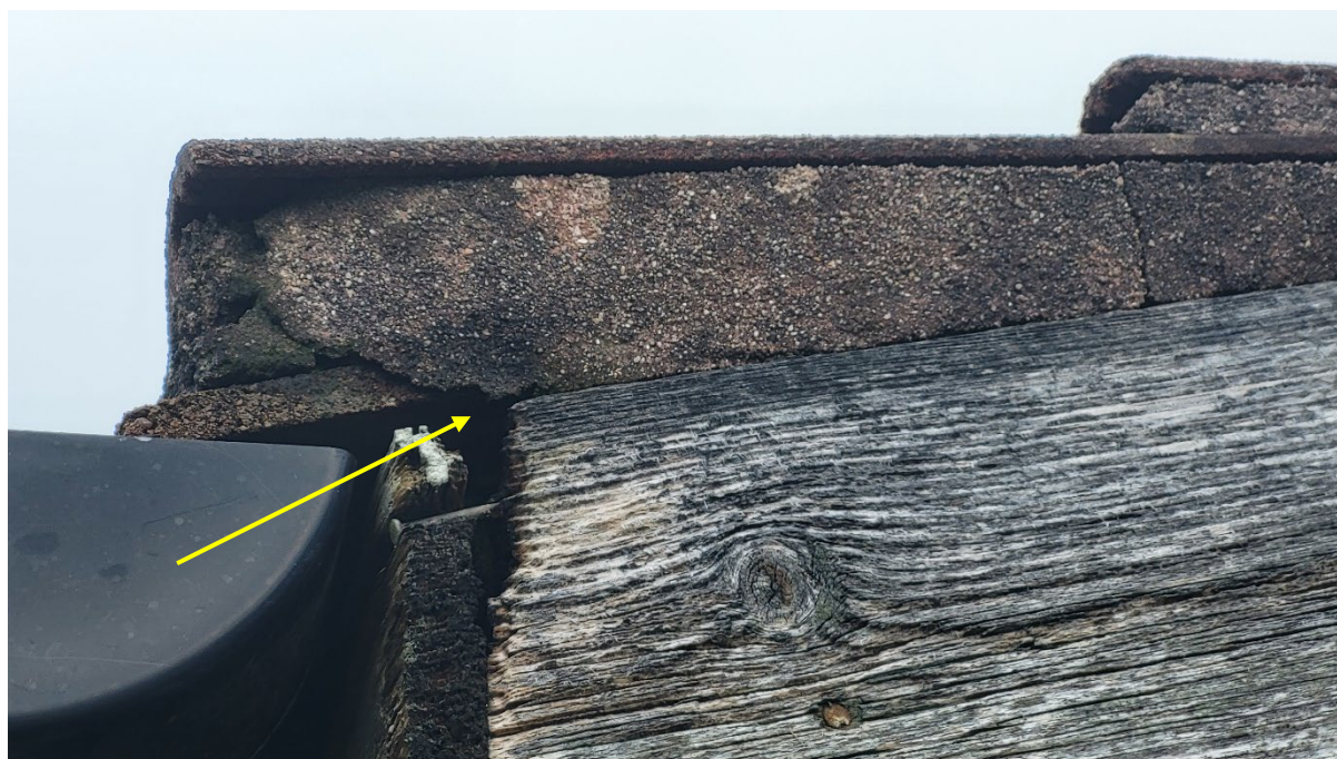
Figure 16: Gap behind fascia on the south-west corner of Racket Town (yellow arrow)
