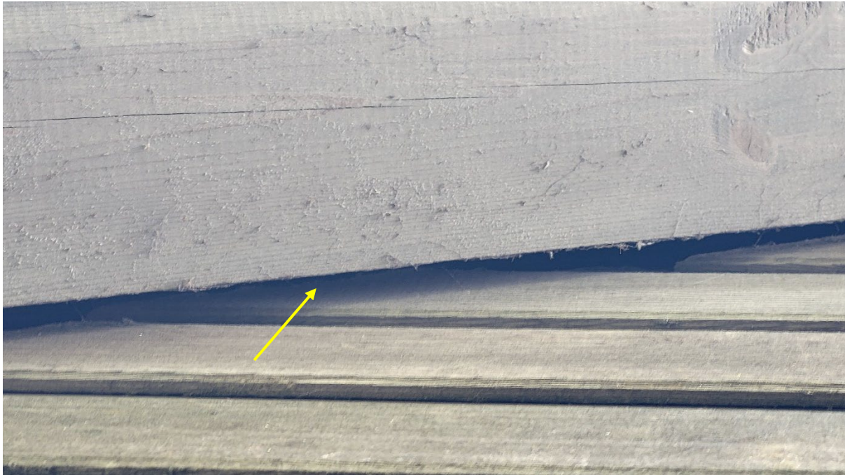
Figure 18: Gap behind soffit on the north elevation allowing potential access for bats (yellow arrow)
