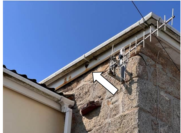
Photograph 2: Showing the gaps behind the fascia on the eastern aspect
