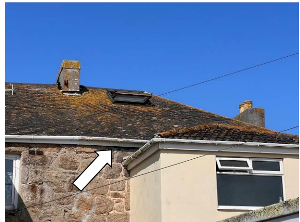
Photograph 4: Showing the gaps behind the fascia on the eastern aspect. The hipped-roof extension is visible on the RHS
