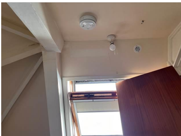
Photograph 5: Showing the top floor accommodation with no apex void
